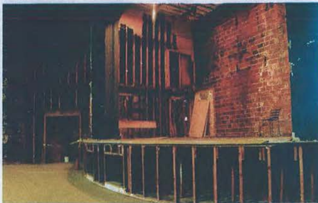
Before the building went into foreclosure, the interior was stripped of nearly all of the remaining decorative elements from the '30s and '50s. Photos by Jesse Wood
